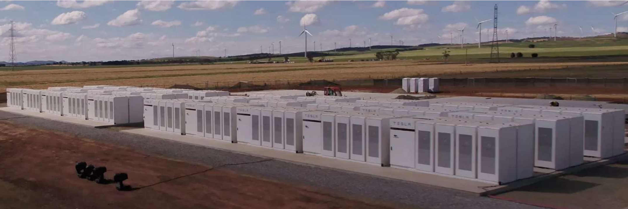
NeoEn-Tesla – 100MWh Battery Storage Plant in South Australia
